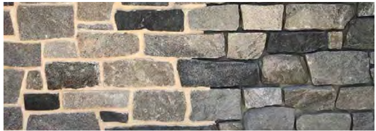
Light vs dark colored mortar joint
